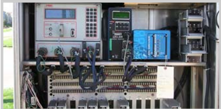
Data collection for signal cabinets and detectors help identify equipment upgrade needs.
